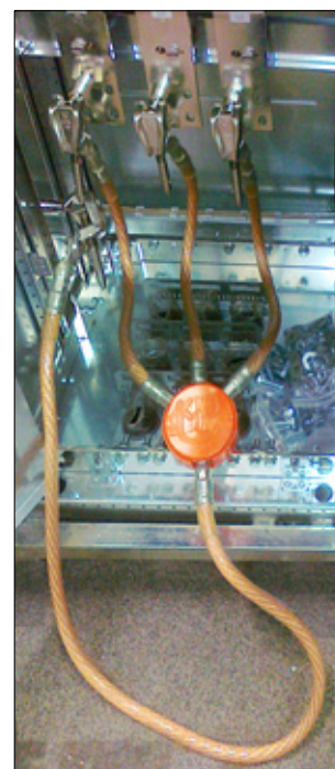
AC busbar grounding
