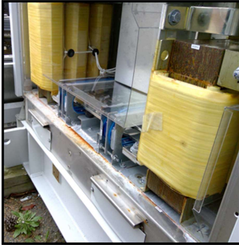
IMAGE 3: Example of premature corrosion
