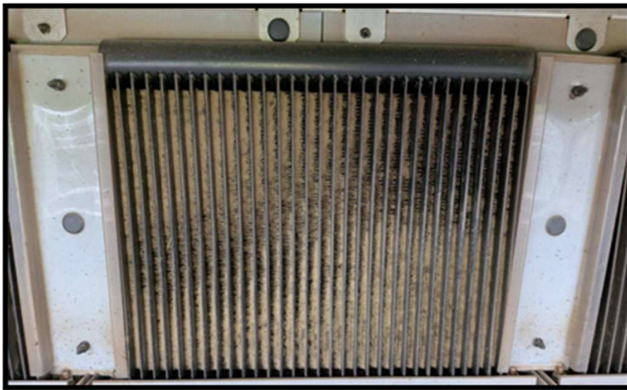
IMAGE 1: Example of filter with excessive debris
