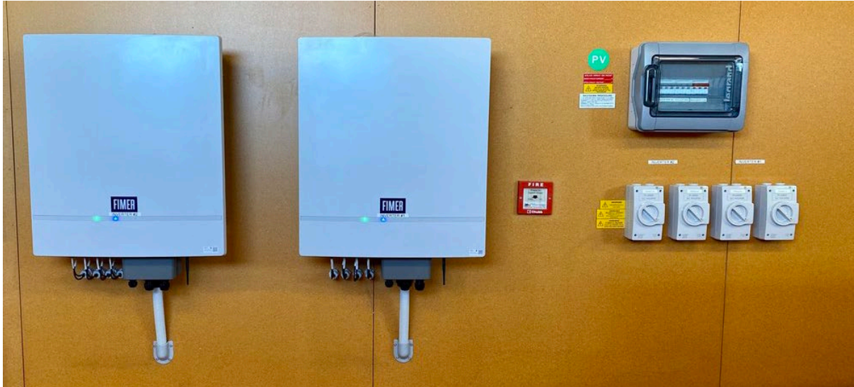
Two of the three FIMER PVS-20 string inverters installed
